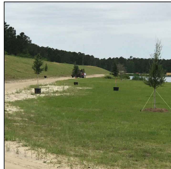
The town is planting trees at the new Town of Awendaw Park and Lake currently under construction.
